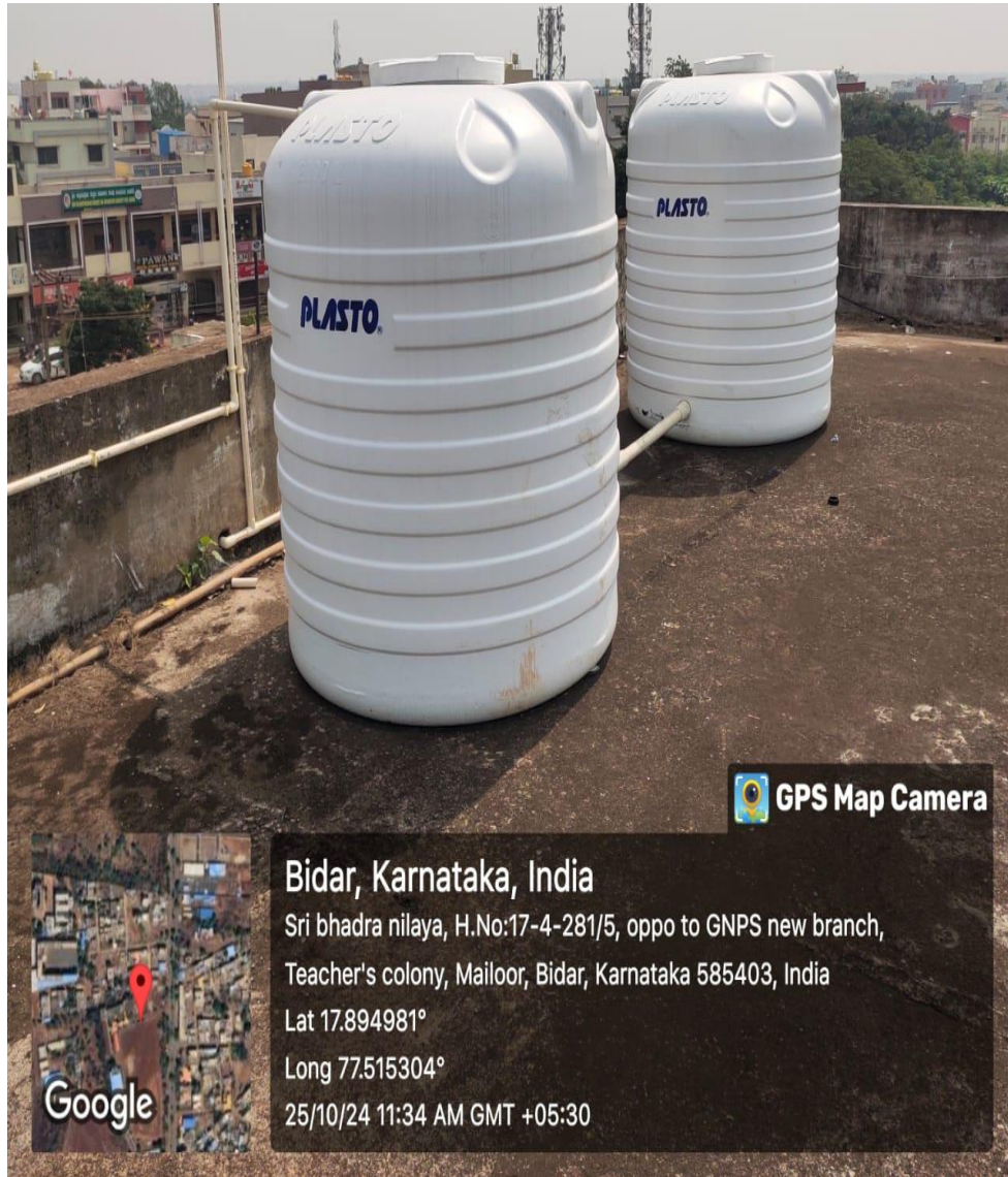
Overhead Tanks in the College Campus
